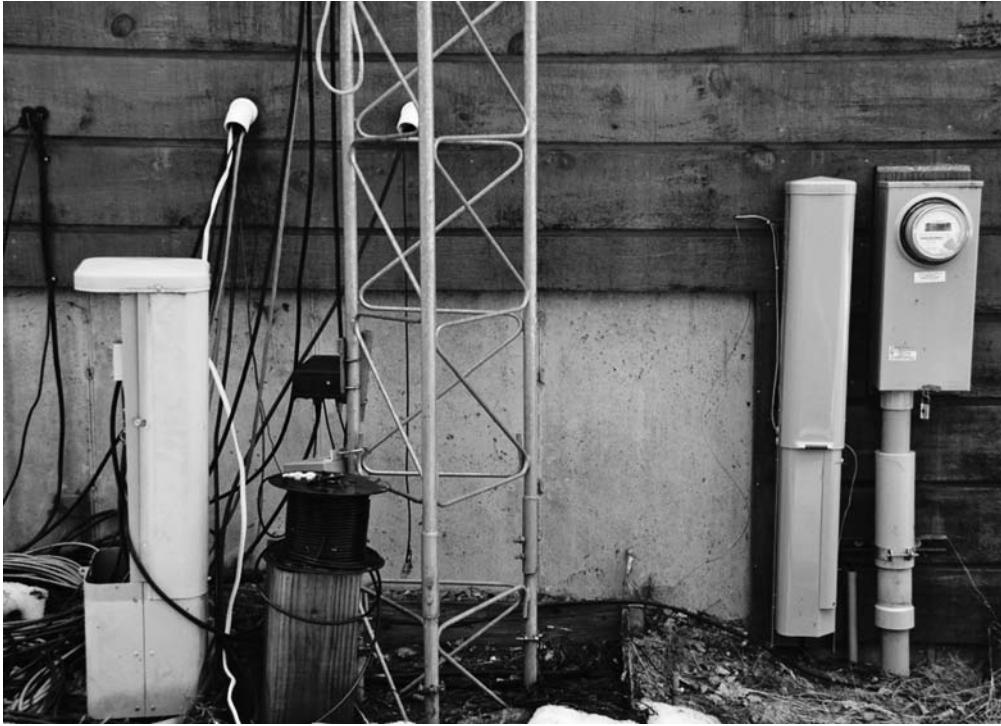
FIGURE 30.2 Single-point ground (SPG) system brings grounds for all utilities, antenna feedlines, and control lines together at a common entry point for the entire building.
